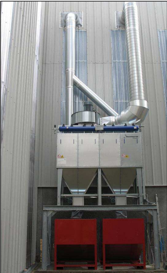
Outdoor installation for block making & pallet brushing stages
