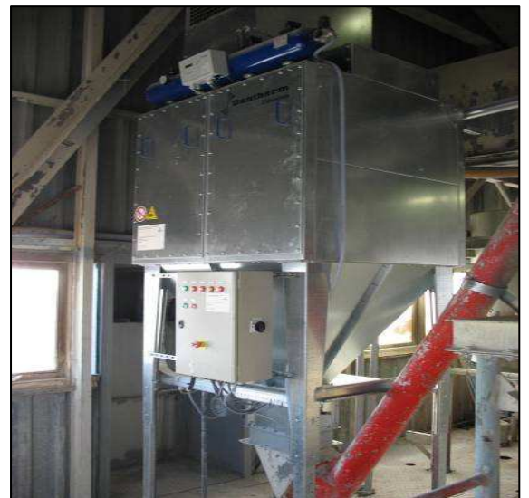
Indoor filter dedicated to a mixing plant
